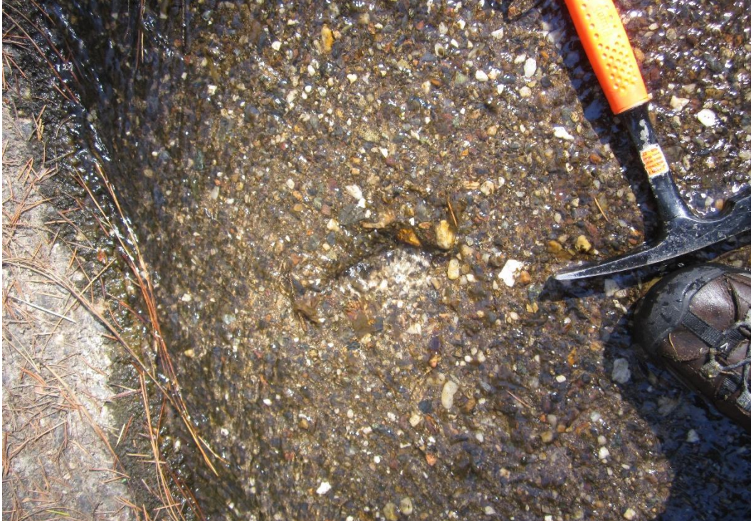
Figure 3-29: Spall upstream of right blanket drain outlet pipe.
