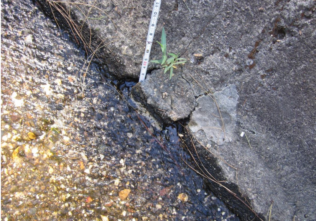
Figure 3-37: Holes in bottom of left side slab at left side of crack 9C.
