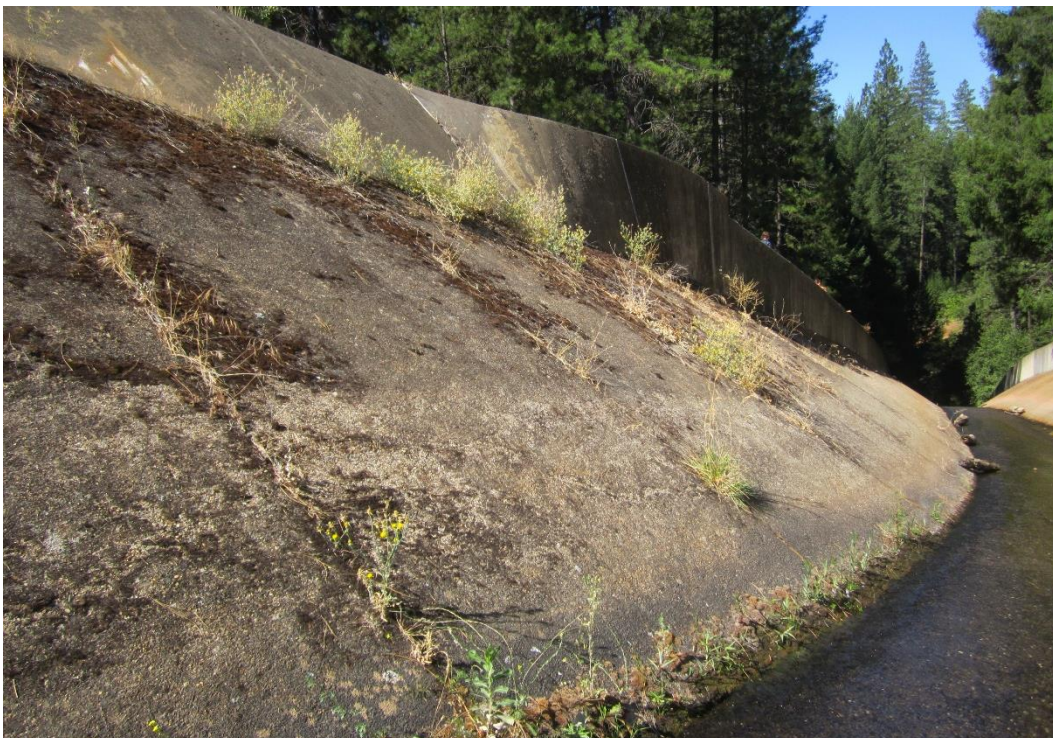
Figure 3-3: Weeds in joints on left side slope slabs.
