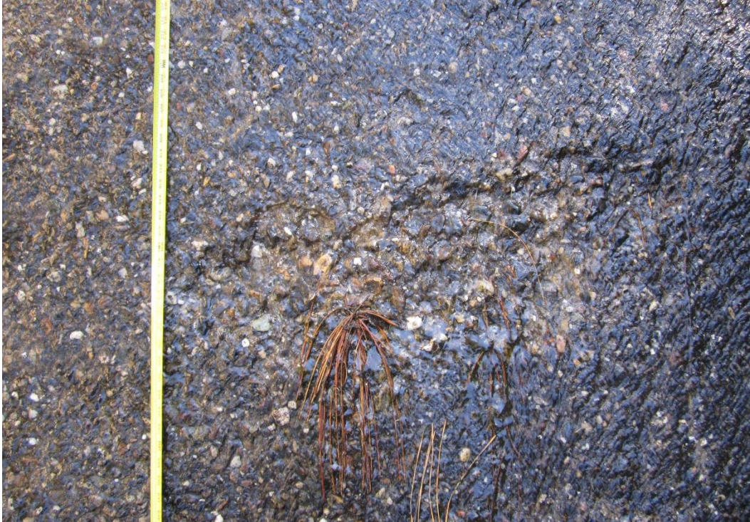
Figure 3-57: Area of deteriorated concrete at 18.5' downstream of Station 5+00.
