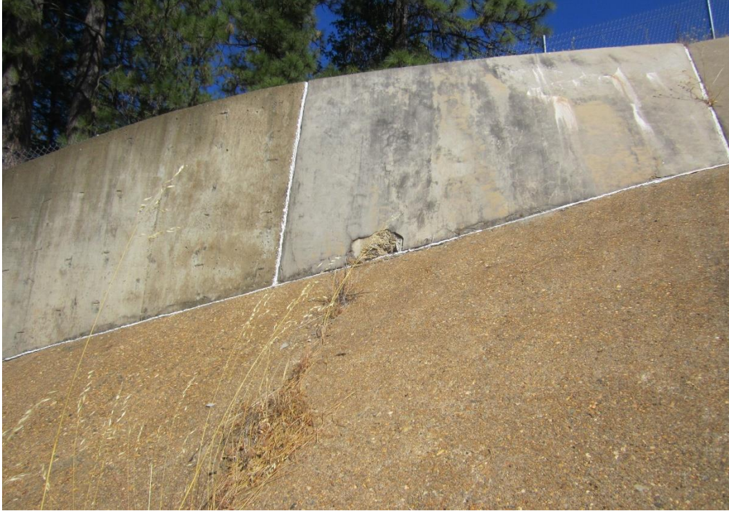
Figure 3-6: Spalled concrete at base of right side slope extension at Station 2+42.
