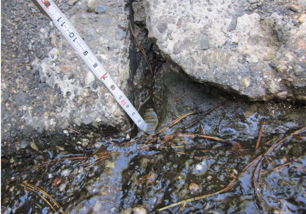
Figure 3-70: Hole at right side of crack 14A.
