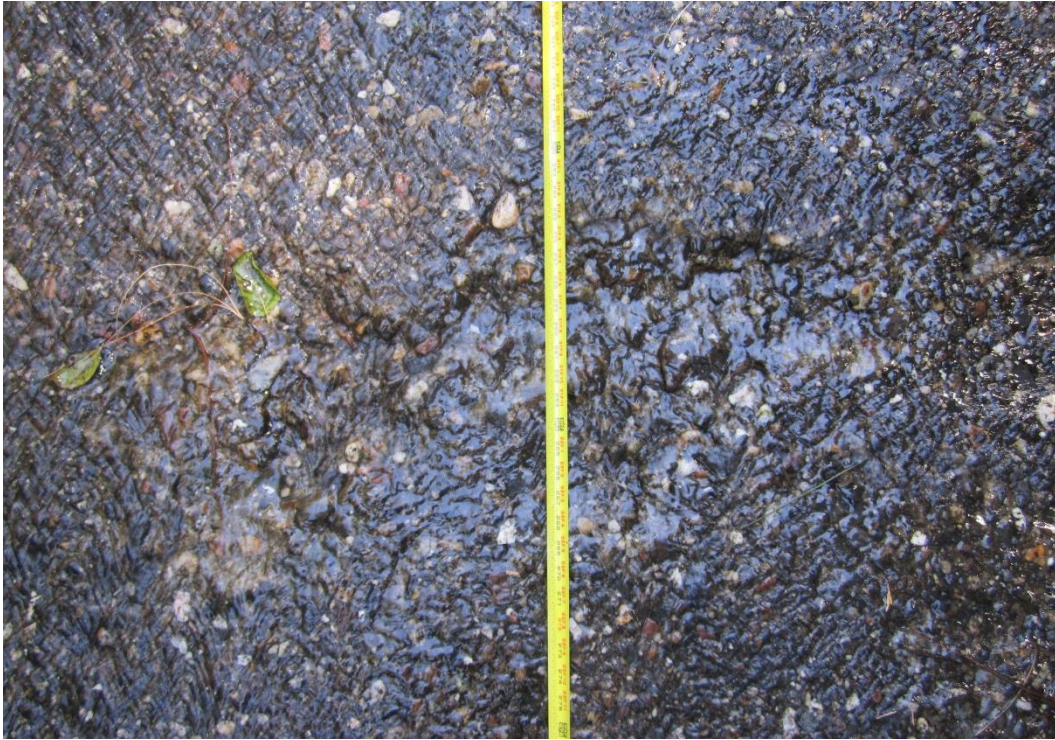
Figure 3-78: Area of deteriorated concrete at 22' downstream of Station 5+75.
