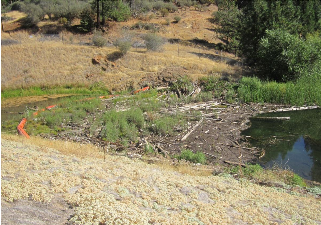
Figure 3-1: Woody debris upstream of log boom across spillway approach channel.
