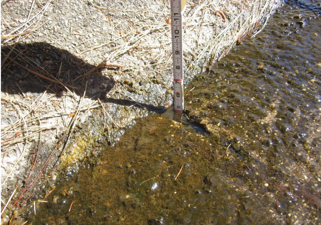
Figure 3-19: Hole in slab at right side of joint at Station 3+25.
