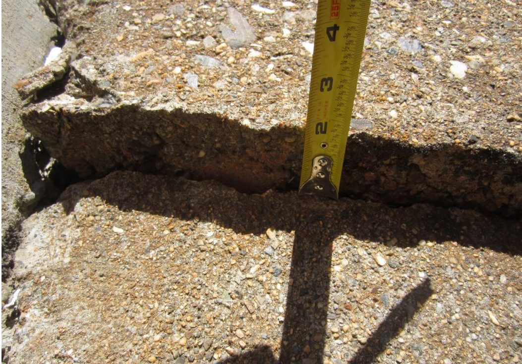
Figure 3-15: Positive offset at top of right side slope slab at Station 3+00.
