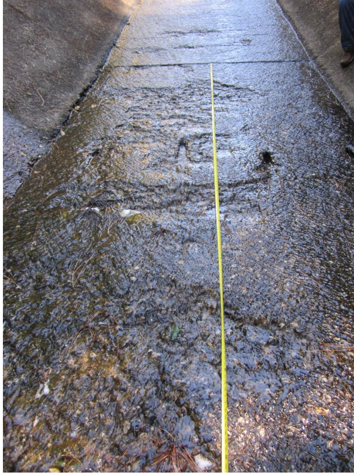
Figure 3-81: Area of deteriorated concrete downstream of Station 6+00.
