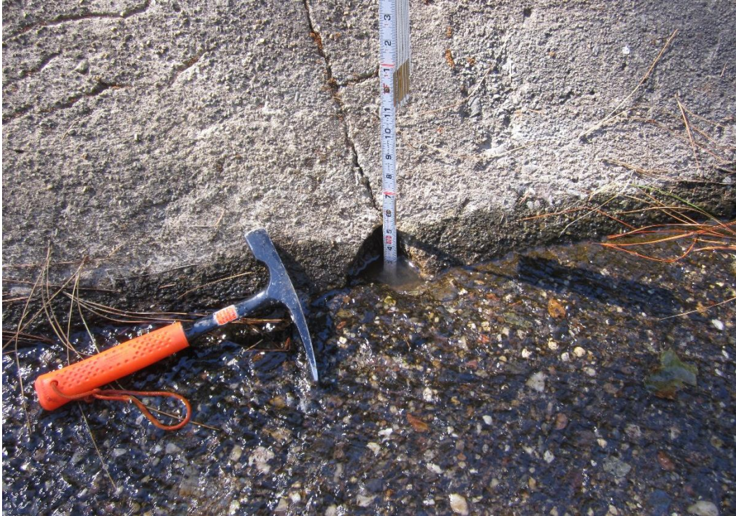
Figure 3-31: Hole in bottom of left side slab at Station 4+00.
