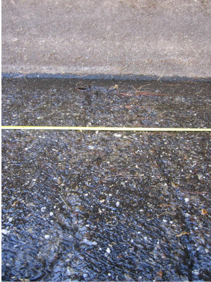
Figure 3-62: Crack 13A and 13B.
