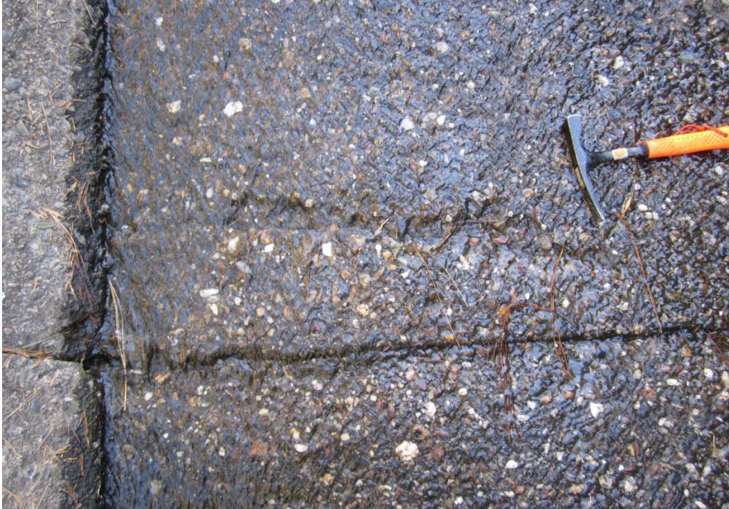
Figure 3-59: Area of deteriorated concrete at 25' downstream of Station 5+00.
